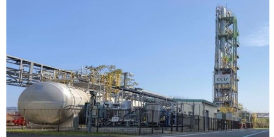
CO 2 separation and capture equipment
